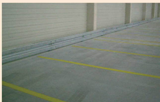
Vangrail B-profiel langs wand
